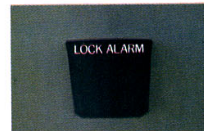
Security Alarm System 21
